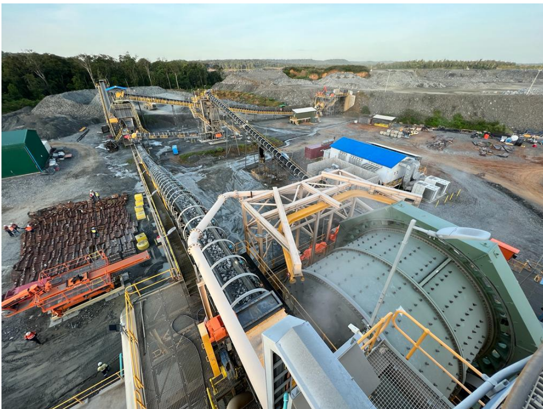
Figure 4 | Okvau Gold Mine Processing Plant July 2022 (SAG Mill Reline Preparation)
