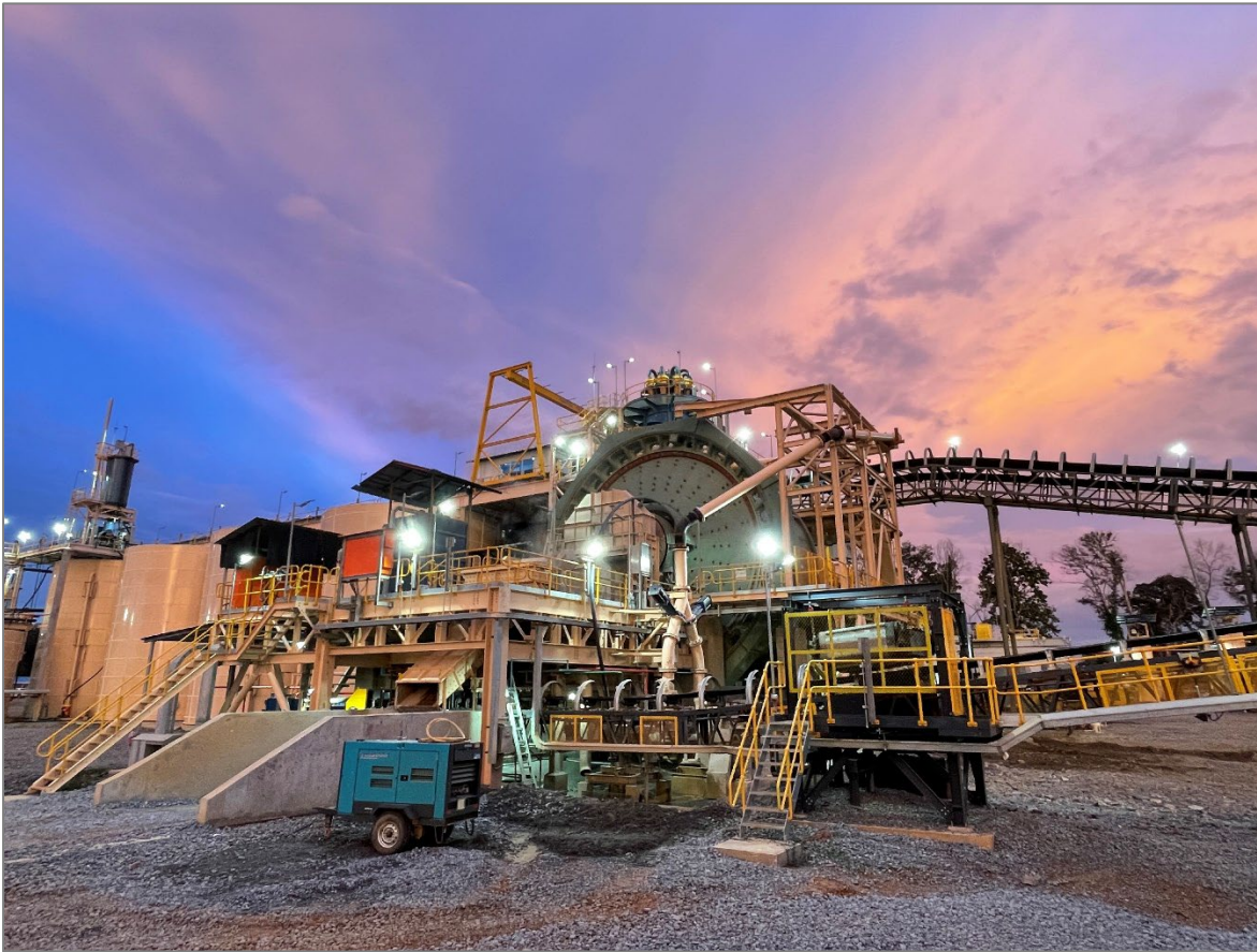
Figure 4 | Okvau Gold Mine processing plant
