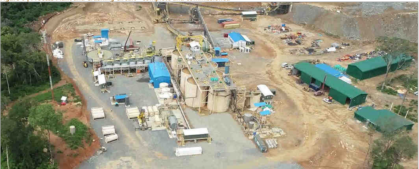
Figure 6 | Process Plant and Crushing Circuit - complete and commissioned
