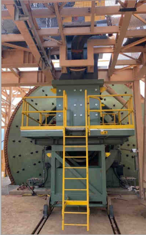
Figure 10 | SAG Mill – commissioned and operating
