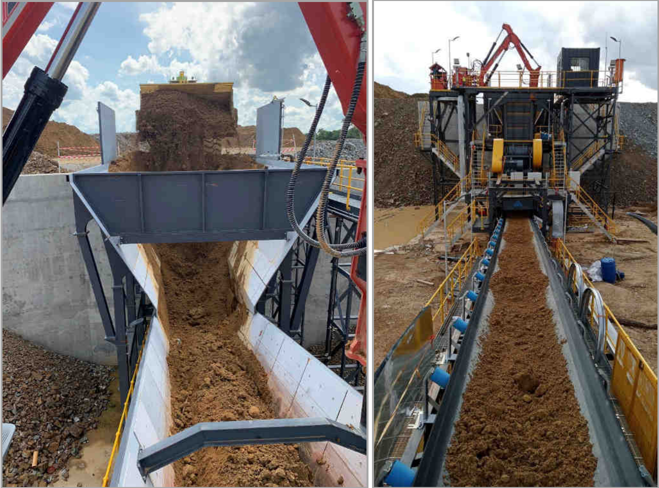
Figure 7 | Crushed ore conveyed to the stockpile
