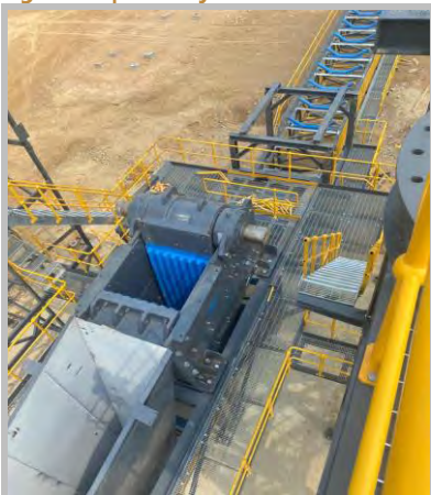
Figure 16 | Primary Crusher Installed
