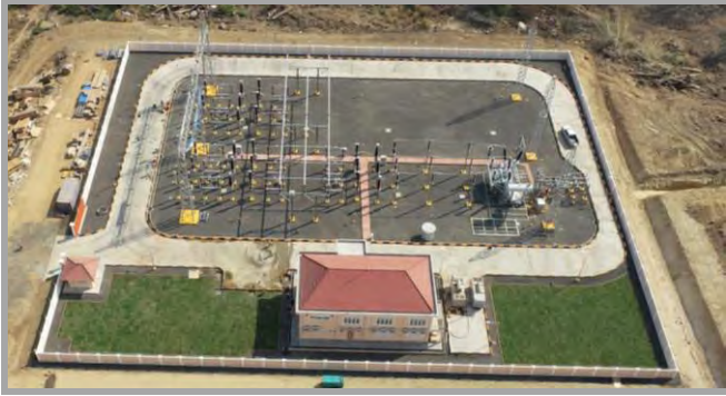
Figure 26 | Substation Aerial Overview
