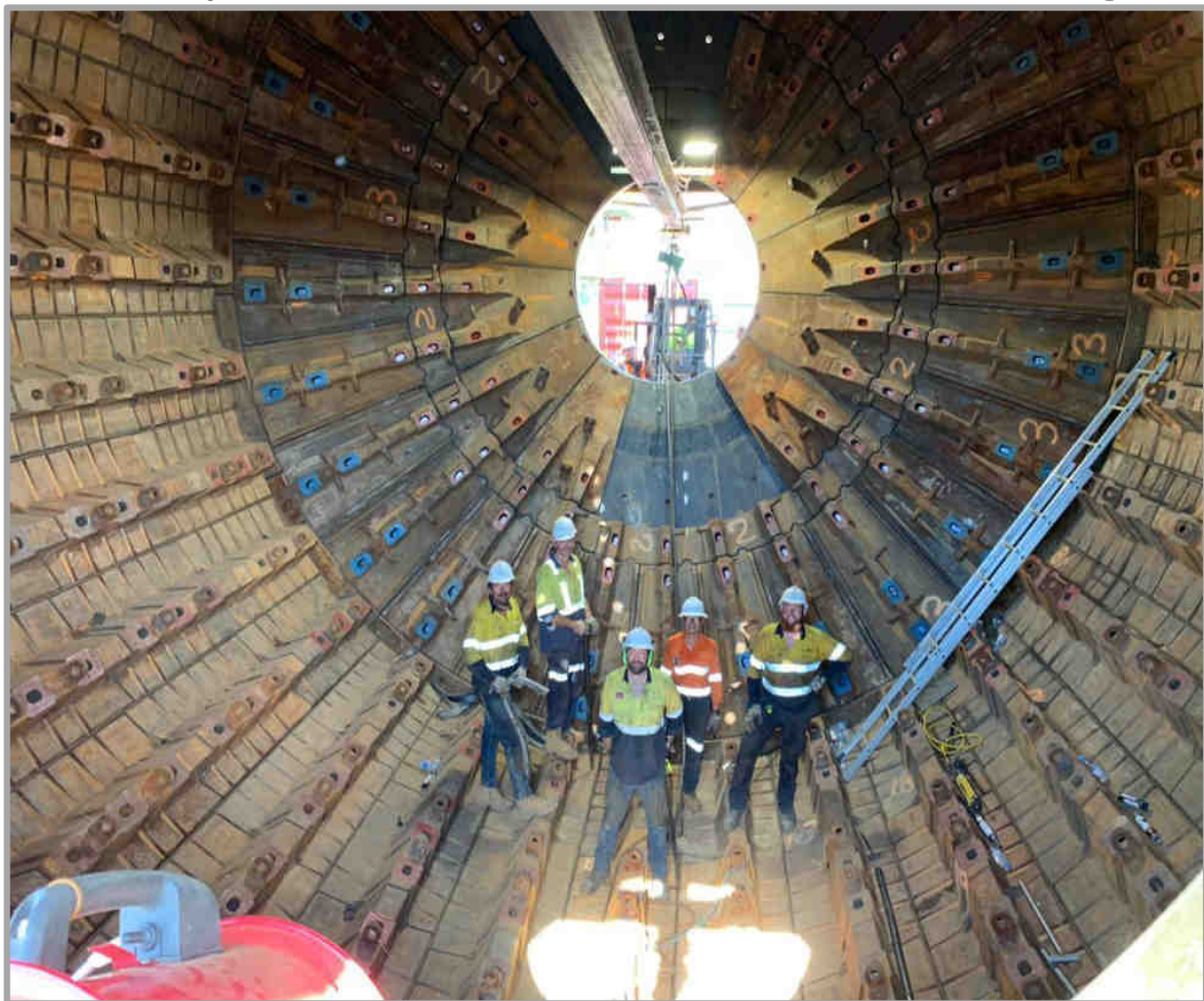
Mill operational management team on site for end of construction and commissioning - stepped in and lined the SAG mill when reline crews unavailable due to Covid-19
