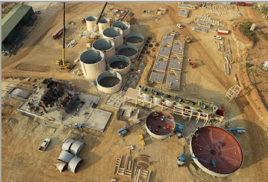
Fig 4: Okvau Processing Plant
