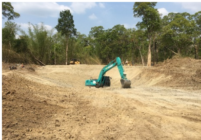
Figure Eleven | Process Plant Sediment Pond
