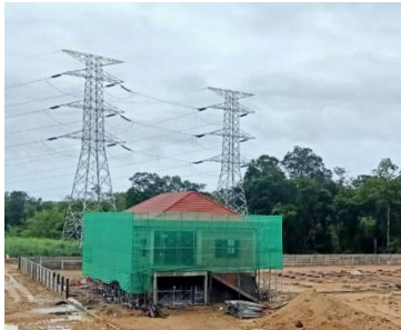
Figure One | Substation Main Control Building
