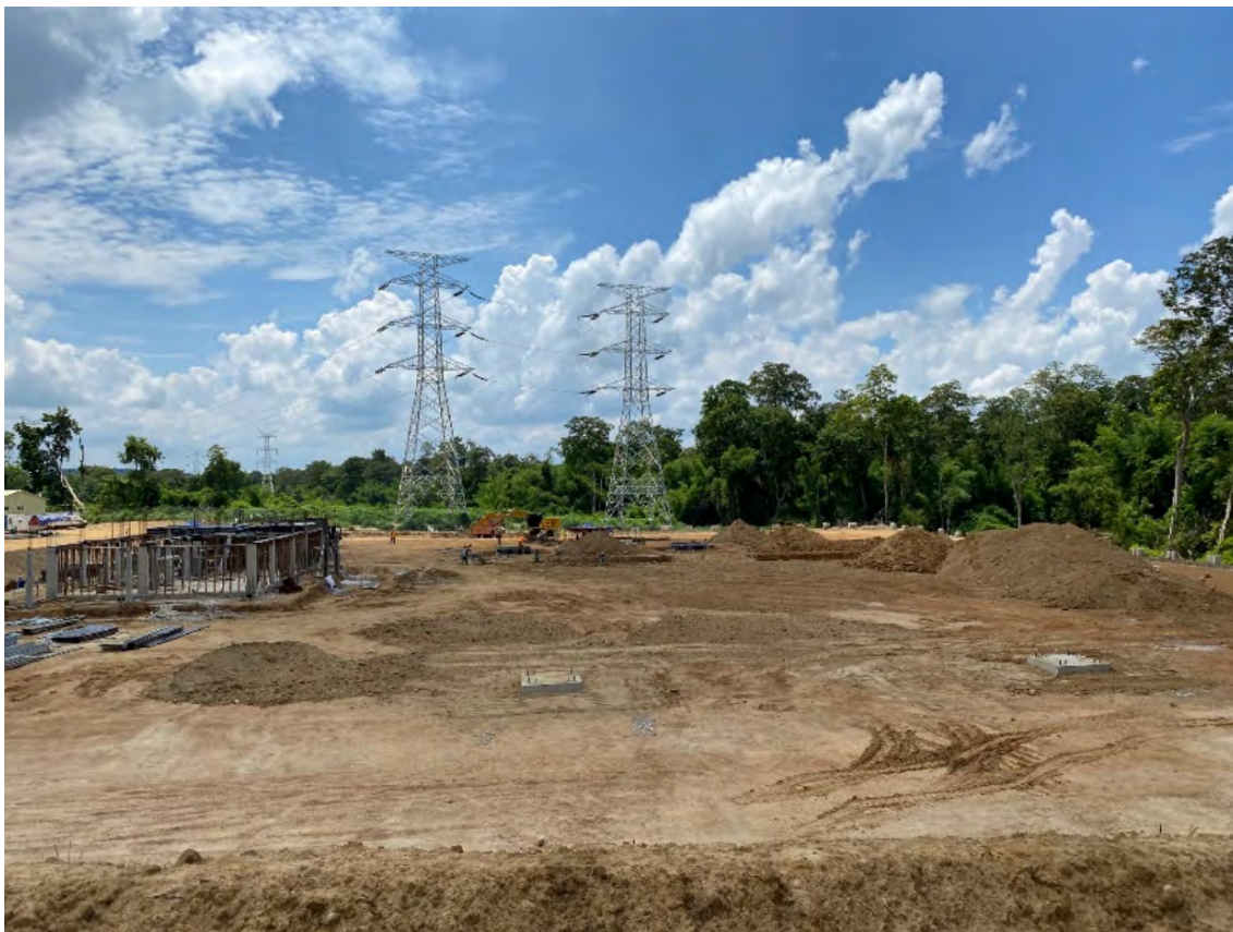
Figure 7 | Substation Control Building area
