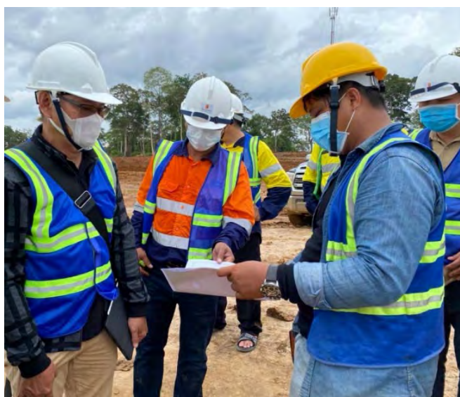
Suitable protocols have been implemented to minimise the potential transmission of COVID-19 while advancing construction activities
