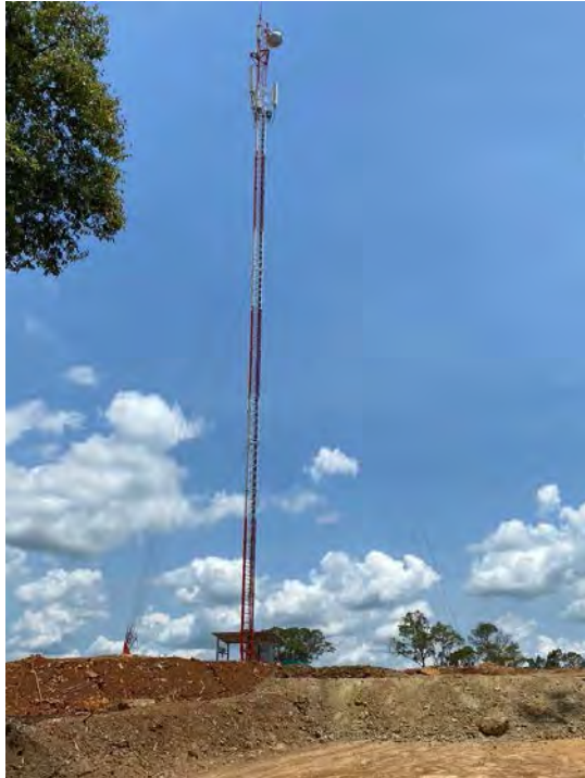
Figure 6 | Site Communications Tower
