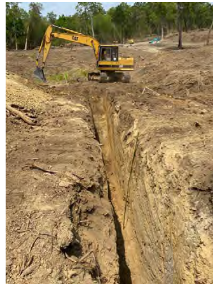
Figure 11 | Plant site cleared and topsoil pushed up following completion of geotechnical stability assessment
