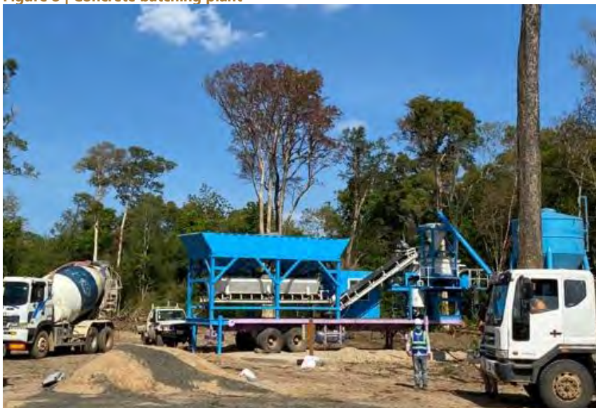
Figure 8 | Concrete batching plant
