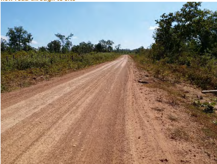
Figure 3 | Okvau Access Road complete which includes substantial upgrades to the existing 50km road and construction of 14km of new road through to site
