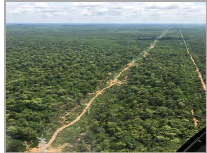
❑ Aerial View Powerline Towers & Corridor nearing completion, and will be available well ahead of site requirements.
